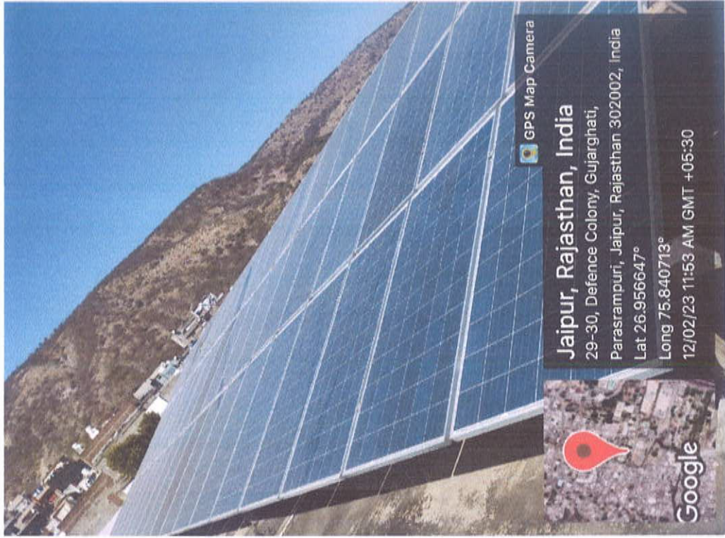
Solar Plant Panel 1
