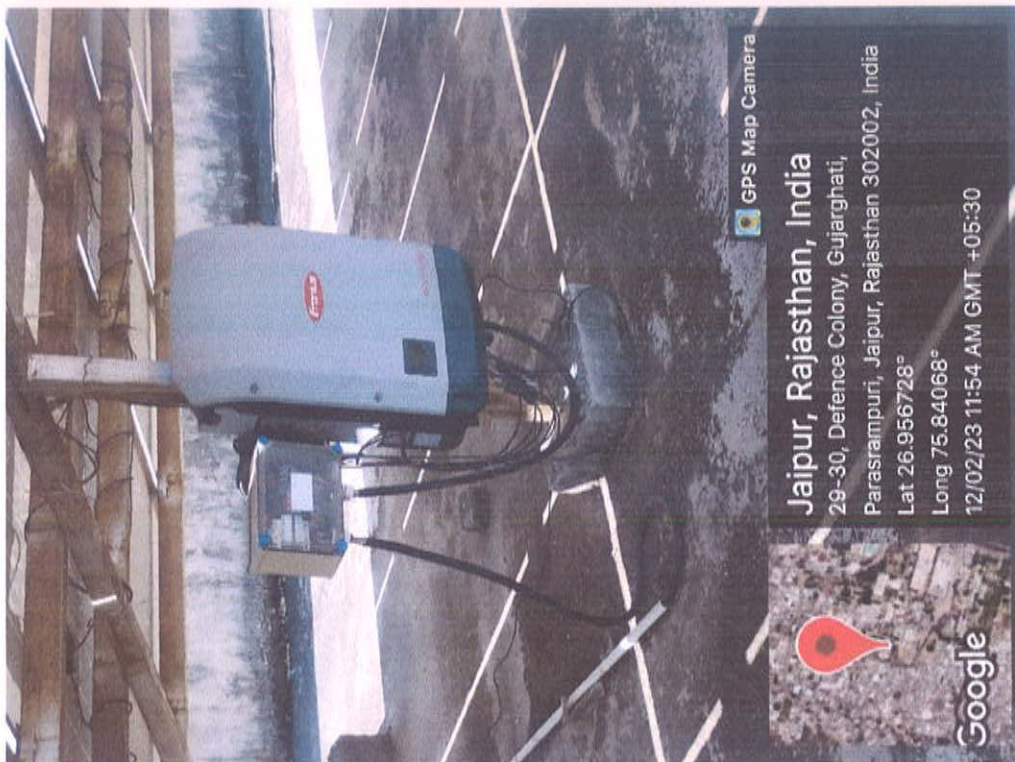
Solar panel power connection
